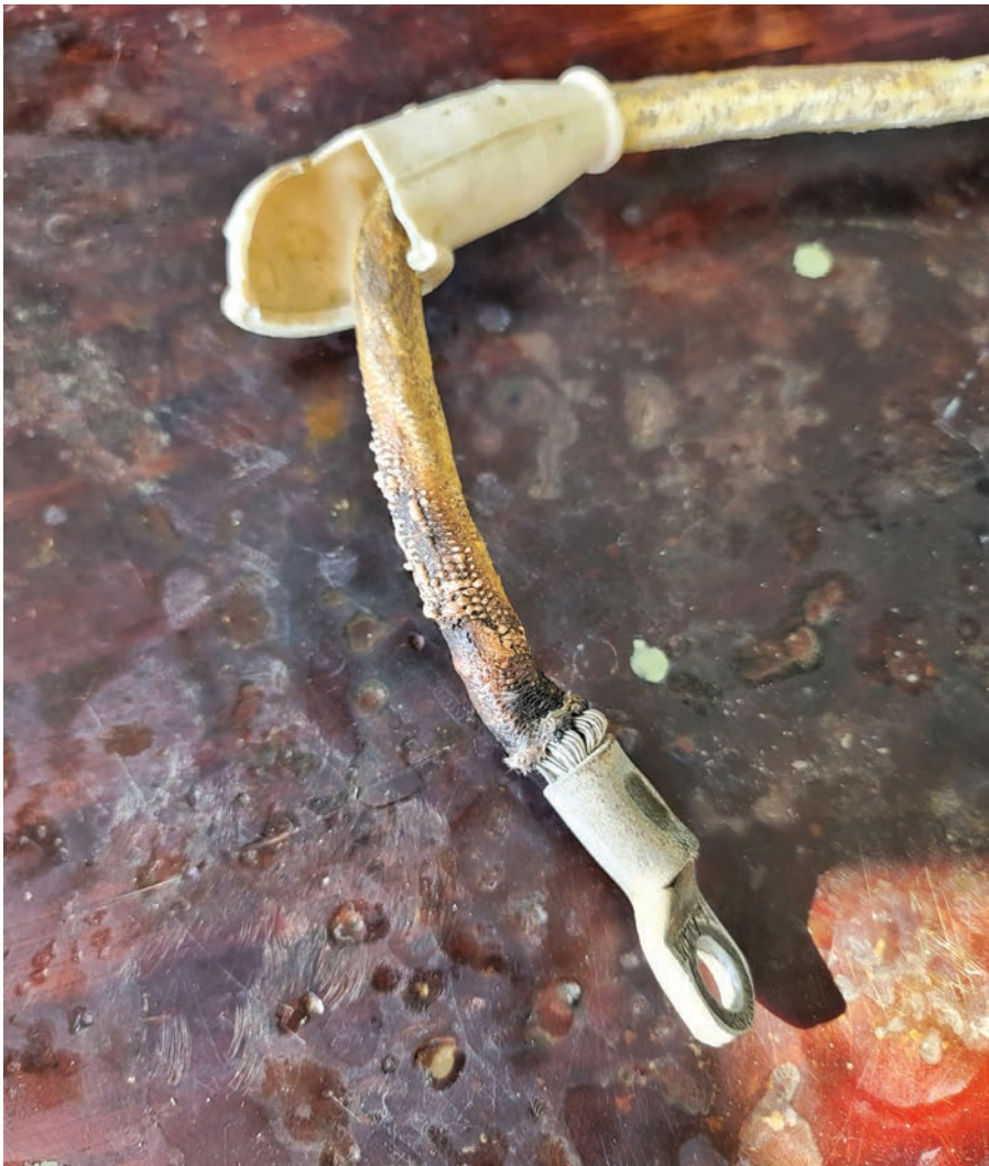
Overheated Battery Cable COURTESY JEN CRIDLEBAUGH
